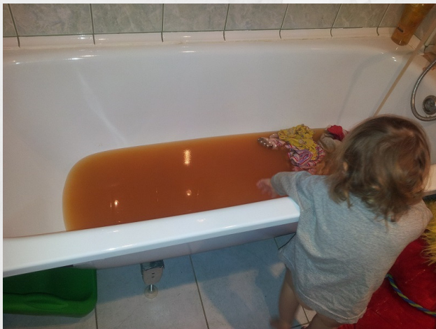
Poor quality of tap water in Pskov region
