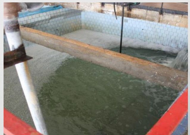
Fine filters of existing water treatment station in Pskov
