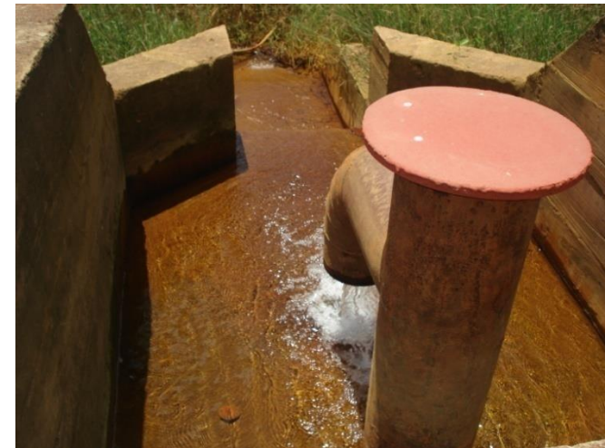
Relief Wells by WAPCOS
