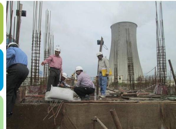
Quality Control Supervision of Kakatiya Thermal Power Project, Stage-II, Warangal, Andhra Pradesh
