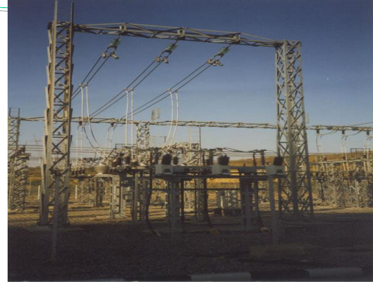
Switch Yard Hwange Thermal Power Station, Zimbabwe
